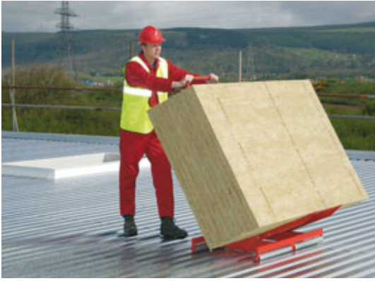
Use of the Rockwool Rock Roller trolley allows fast and easy movement of boards across the roof decking
