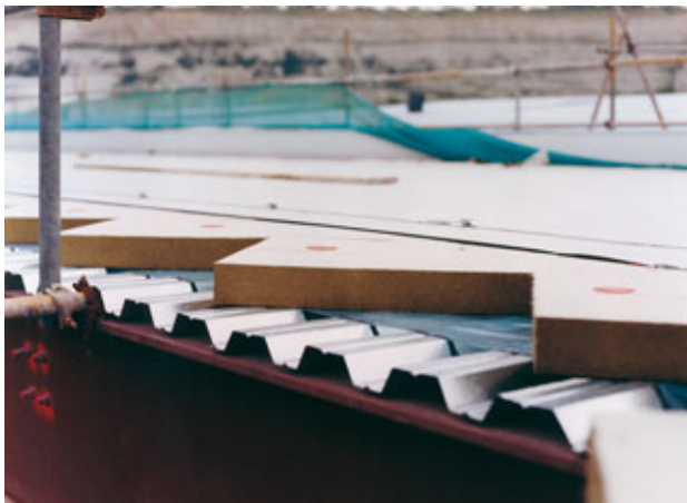
Hardrock Dual Density roofing boards applied below mechanically fastened single ply membrane.
